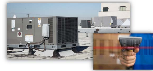
Figure 66: RFID Tagging Equipment
